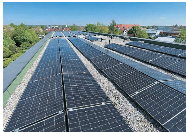
Solar panels on the roof
